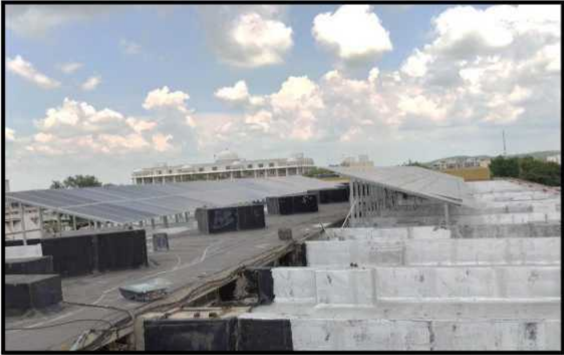
Solar panels system to provide uninterrupted power supply for ICT tools and infrastructure
