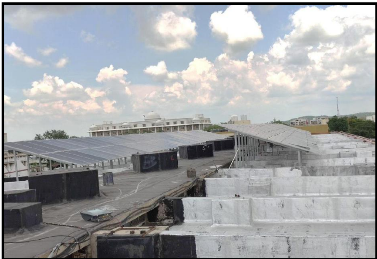
Solar panels system to provide eco-friendly power supply for ICT tools and infrastructure
