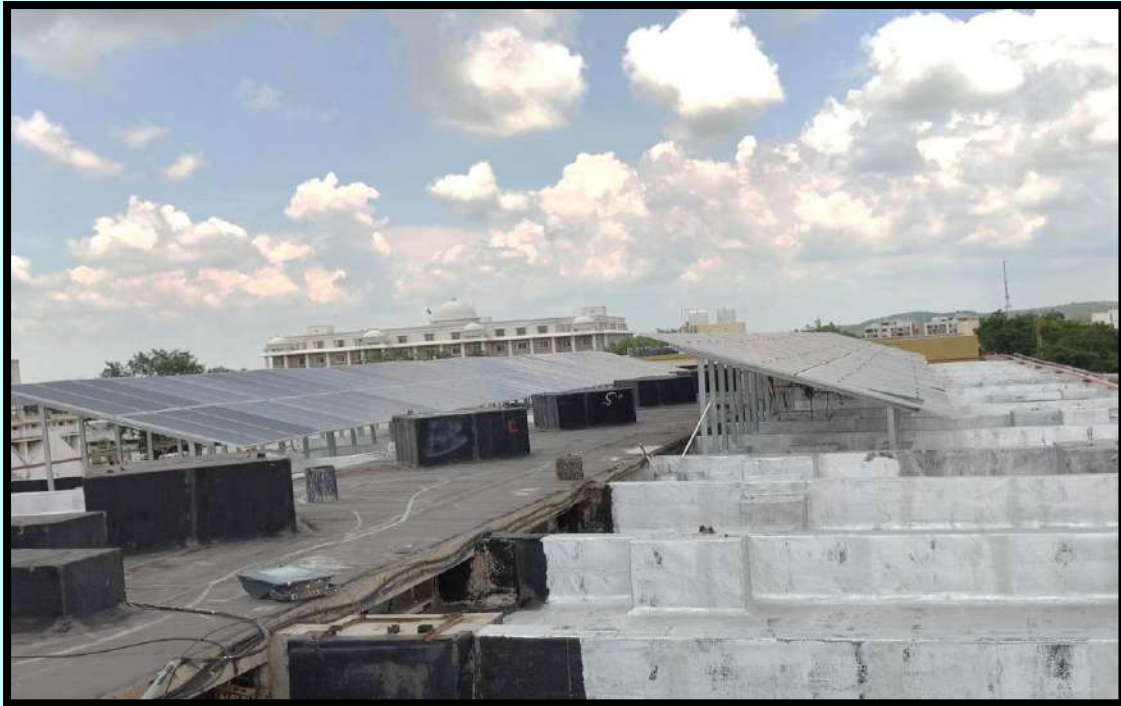
Solar panels system to provide uninterrupted power supply for ICT tools and infrastructure
