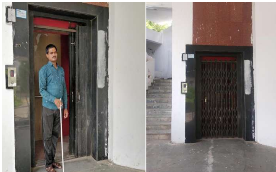
Elevator in Main Building
