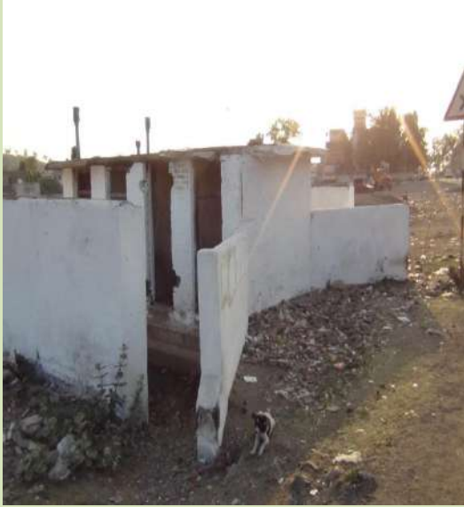
Damaged Toilets, Adarsh Nehru Nagar Amt
